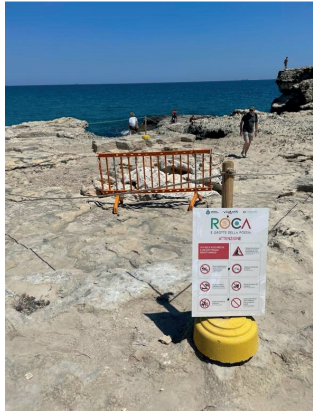
Figure 4 : Above part of the karst system, open cracks at the surface indicate the high risk of further collapses.
